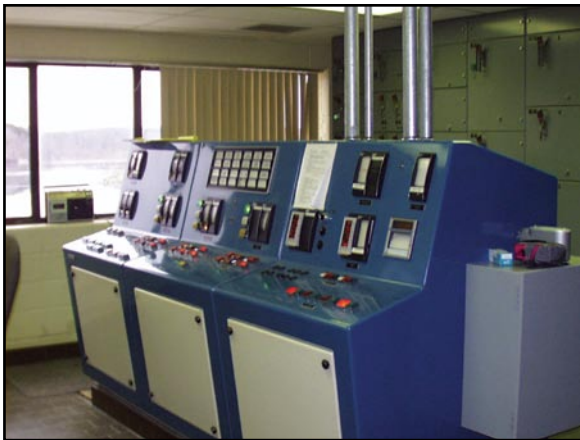
The old 1977 'state of the art' plant control panel
