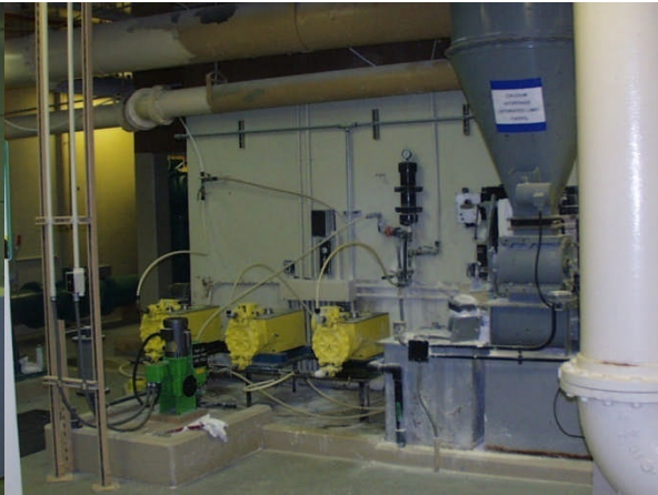
Lime Feed- Original 1978 Equipment
