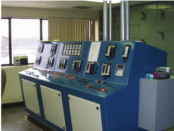
Outdated 1978 Control Panel
